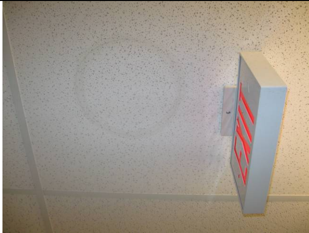
PHOTO 1 – STAINED CEILING TILE – HALLWAY BY CENTER ENTRANCE TO SCHOOL.
