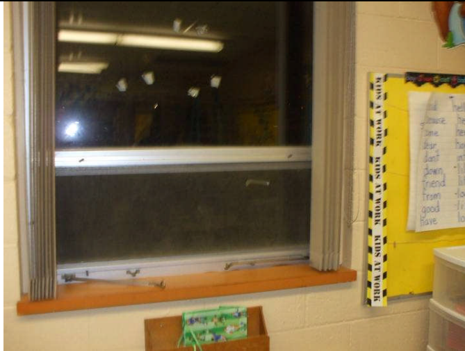
PHOTO 1 – ROOM 109 – EXAMPLE OF WINDOW SCREEN WITH VISIBLE DUST.
