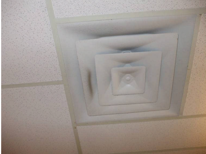
PHOTO 5 – EXAMPLE OF HVAC AIR SUPPLY DIFFUSER SHOWING DUST BUILD UP.
