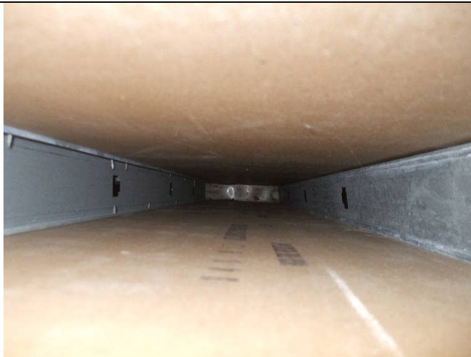
PHOTO 3 – AN EXAMPLE OF AN AREA OF DRYWALL WALL INSPECTION BETWEEN ROOMS 109 AND 107 – PHOTO TAKEN FROM ABOVE CEILING TILE LOOKING DOWN.
